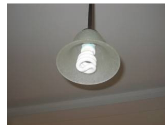
Compact fluorescent lamps are used in the
