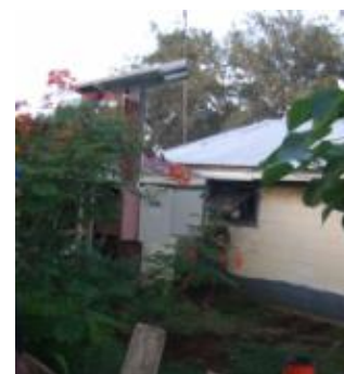
Recently installed solar system on Mango Island
