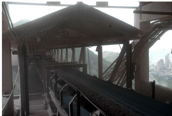
Covered Conveyors, but emissions fugitive ©ACC Ltd
