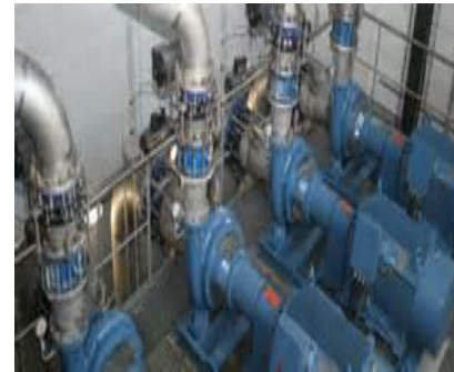
Pumping station CRDA
